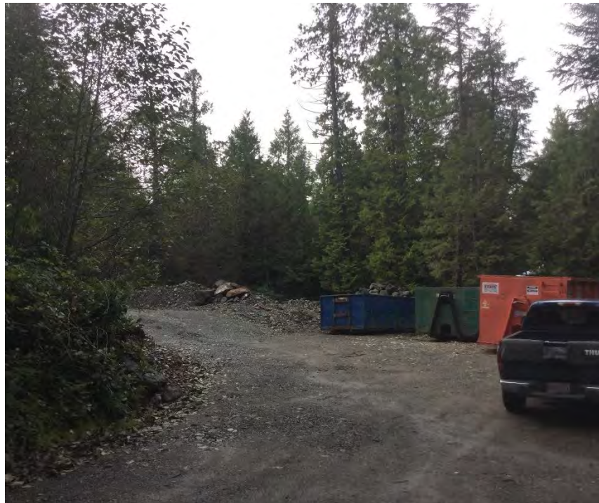
Photo 1. The subject property as seen from the driveway access off Peninsula Road. The lot has been partially cleared of trees to support the creation of a gravel access road.
